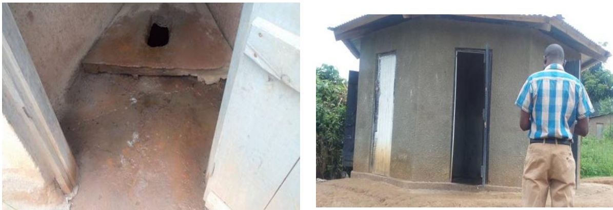
Figure 8: Boys latrines without hand washing containers
